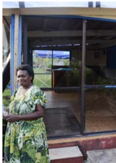
Enikelen Netine outside the PWMU Project House in Port Vila. It lost its roof and suffered significant damage.
